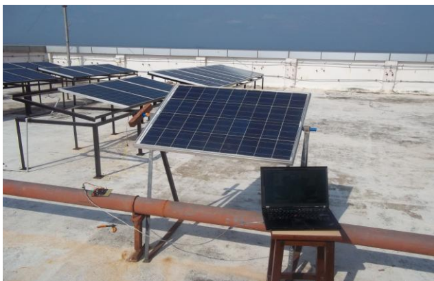
Figure 4. Tracking system installed in a solar panel.
